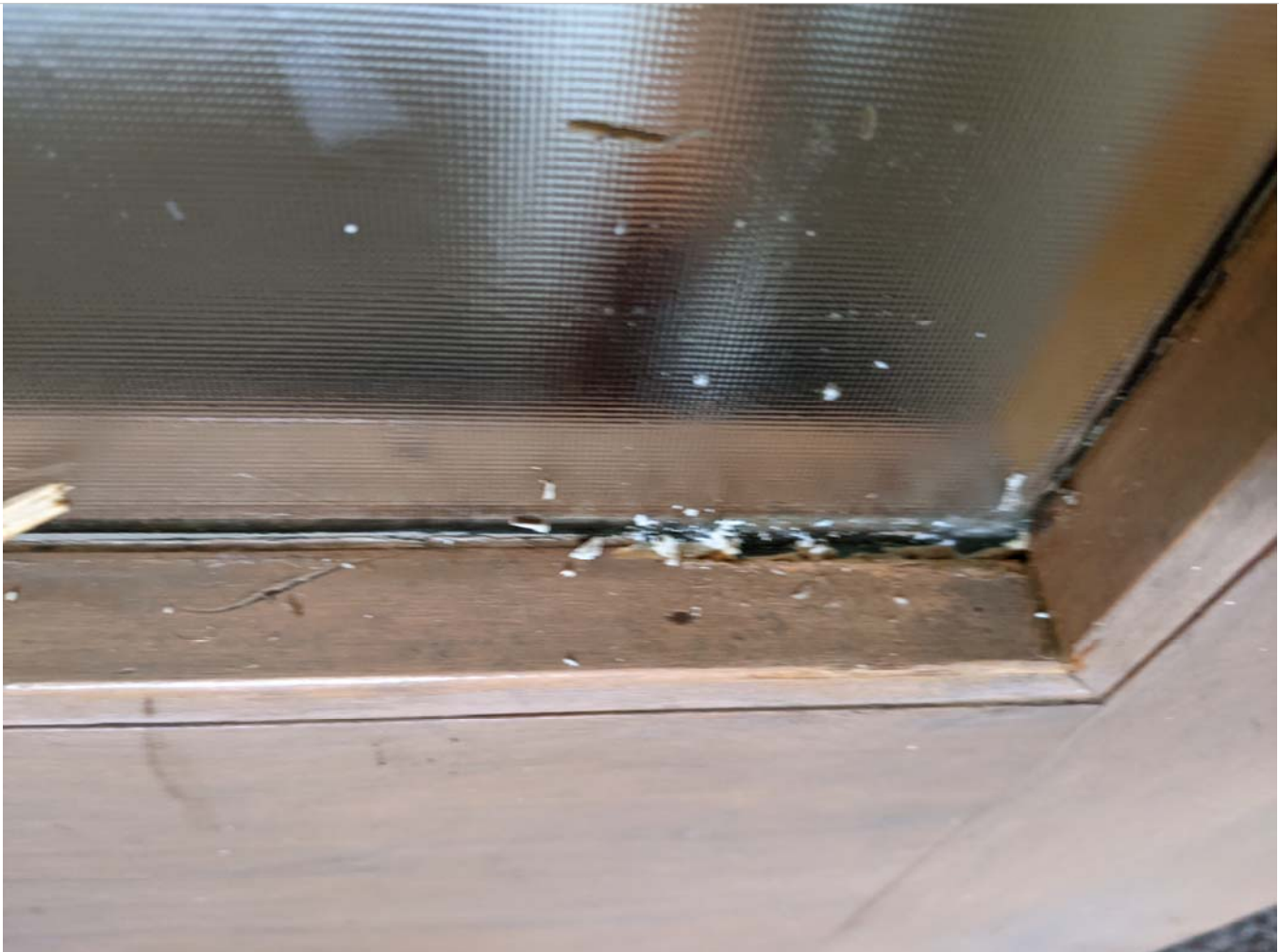
ACM glazing in door-typical
