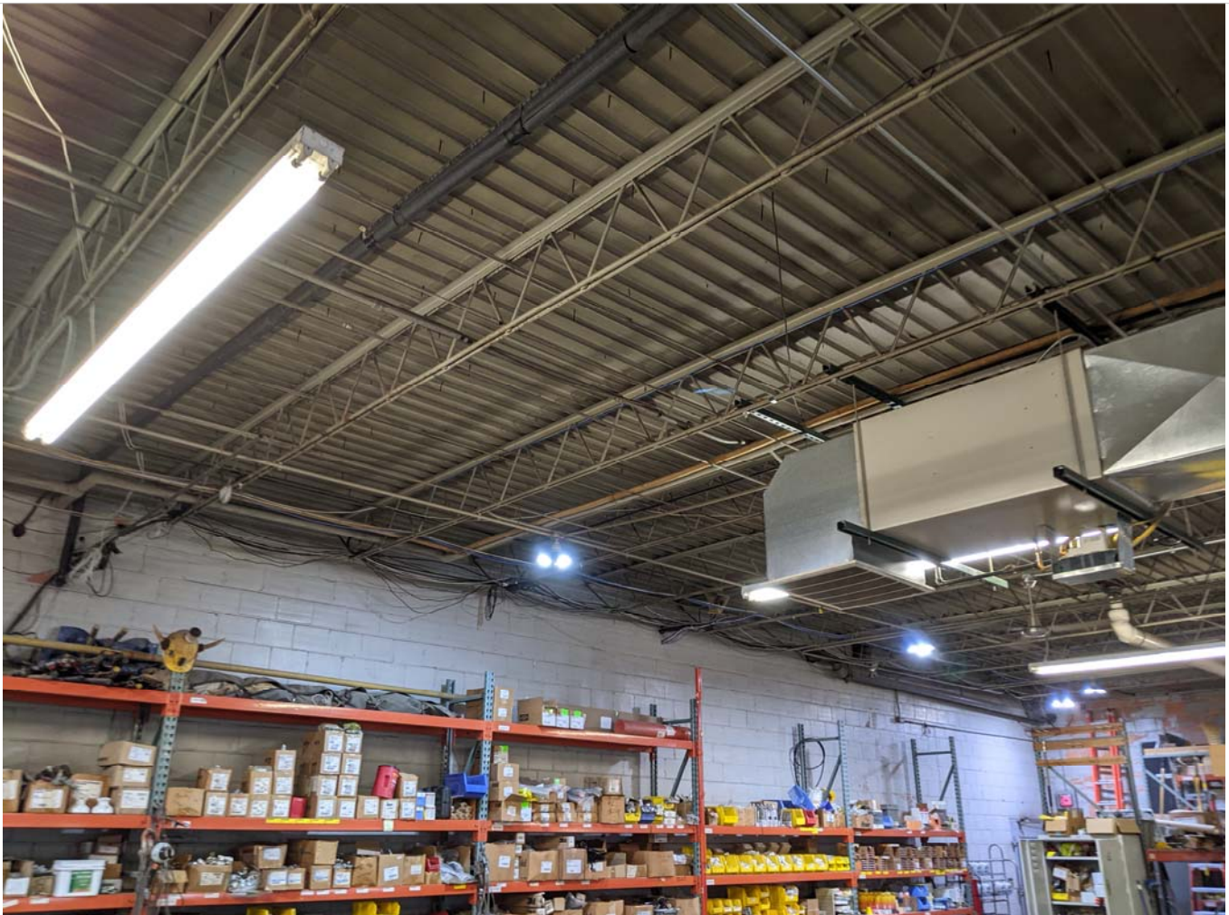
ACM pipe insulation-garage-typical
