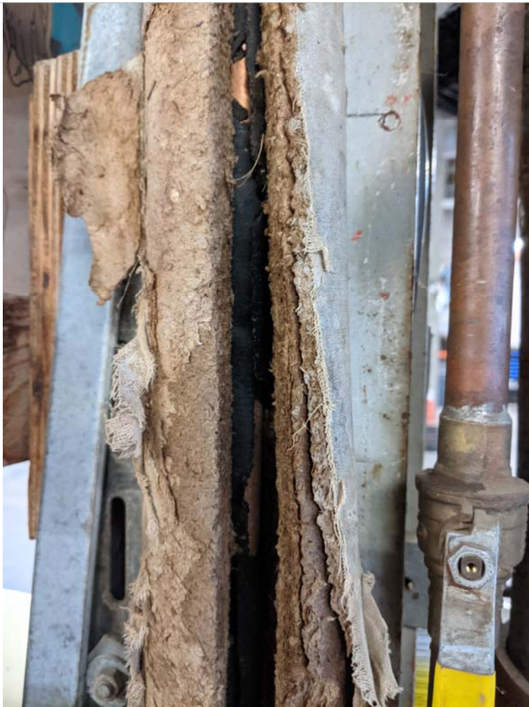
ACM pipe insulation-inner black paper layer-typical
