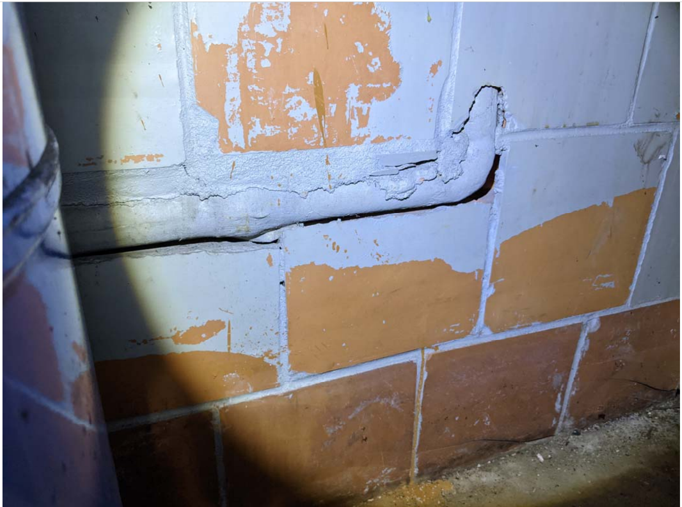
ACM pipe insulation in wall cavities
