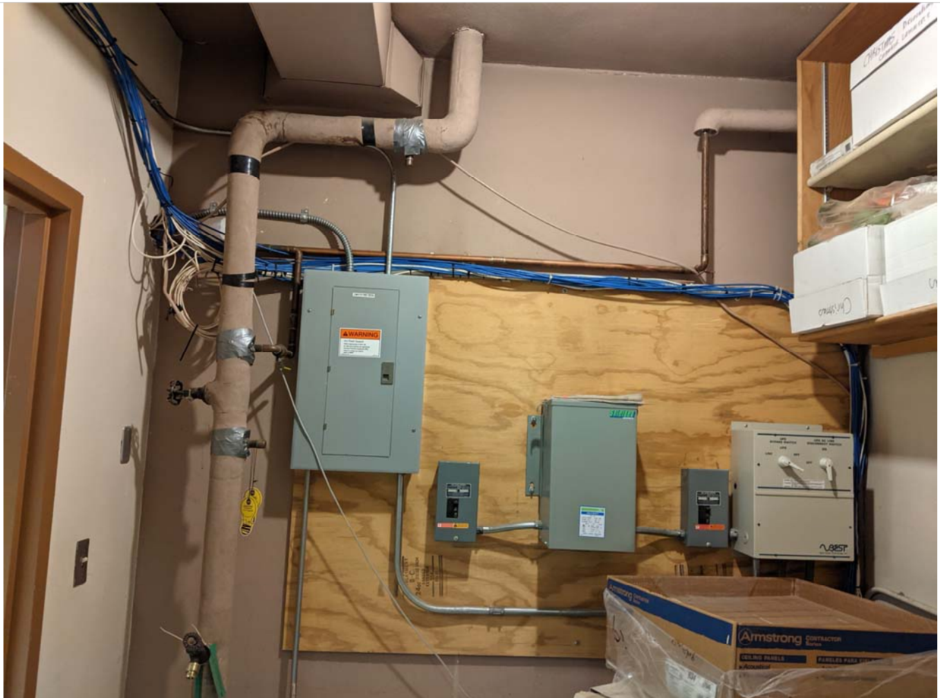
ACM pipe insulation-typical
