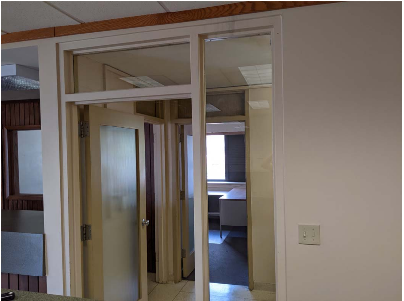
ACM glazing in door and window-lobby
