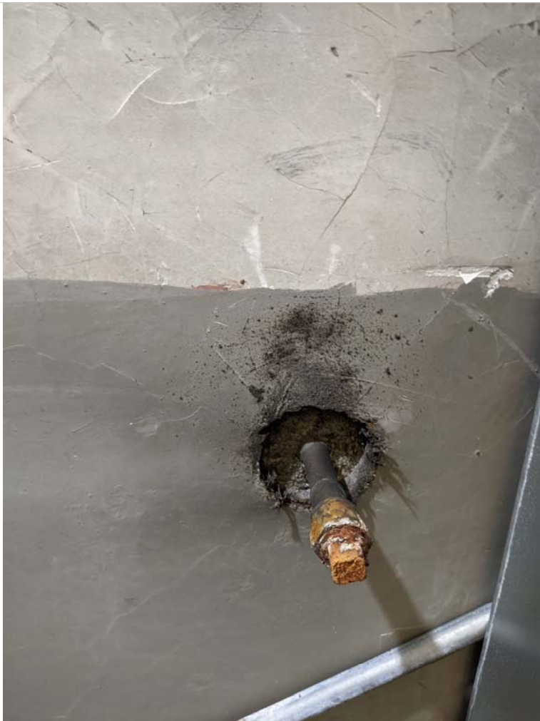
ACM pipe insulation in ceiling- Equipment room
