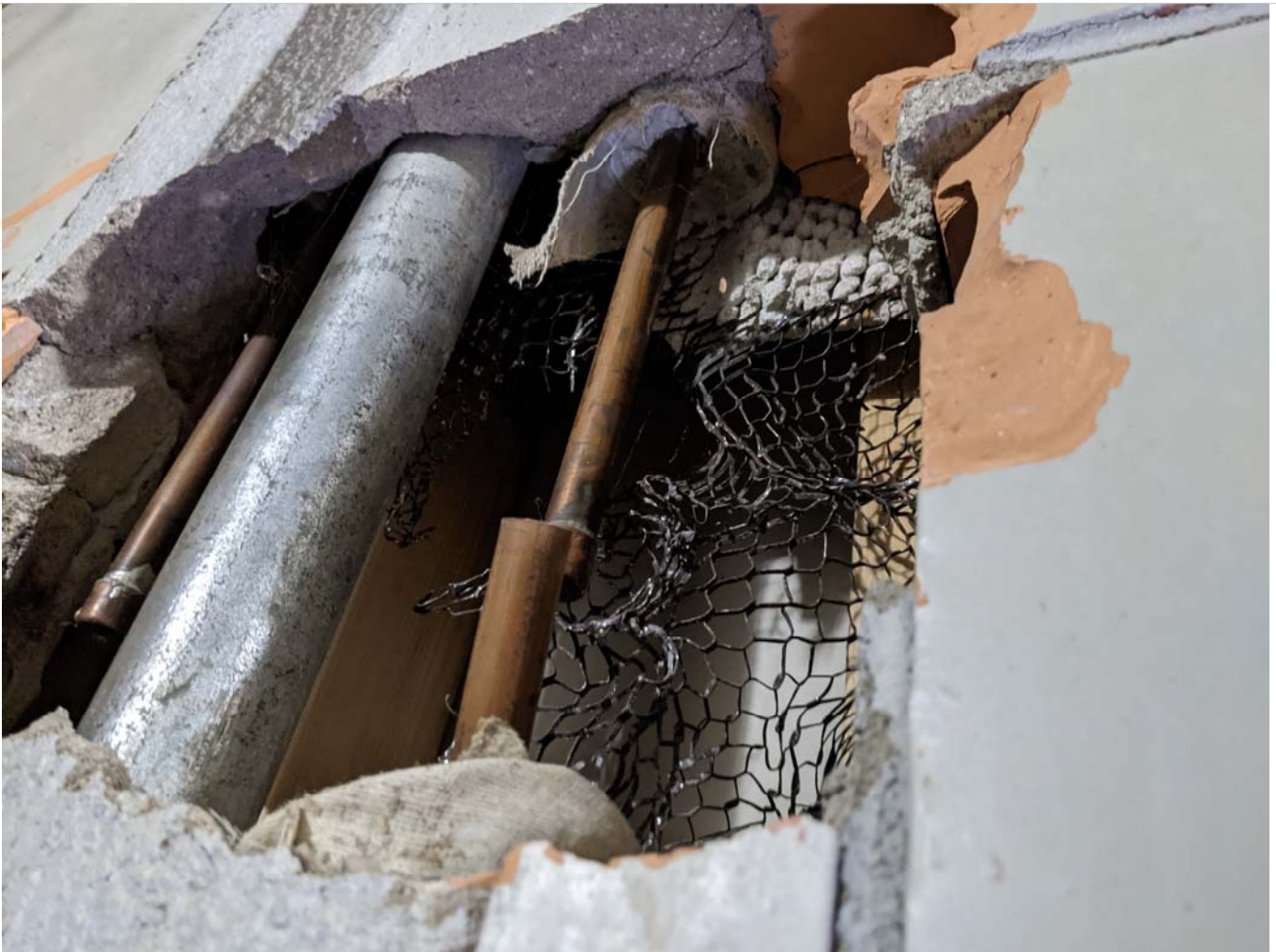
ACM pipe insulation in wall cavities
